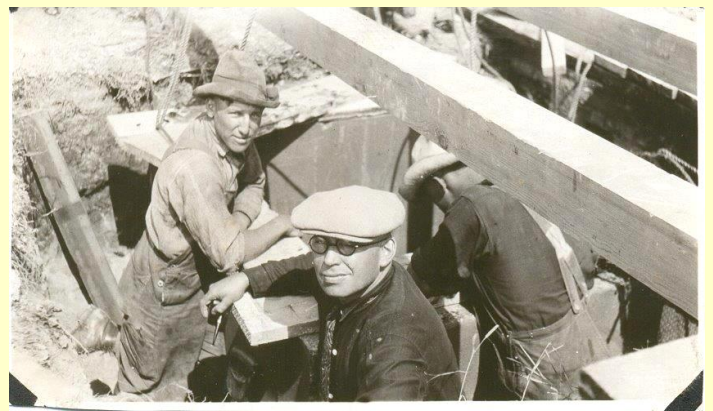
Clarence Anderson and Paul Goering capping the flour mill well after demolition
