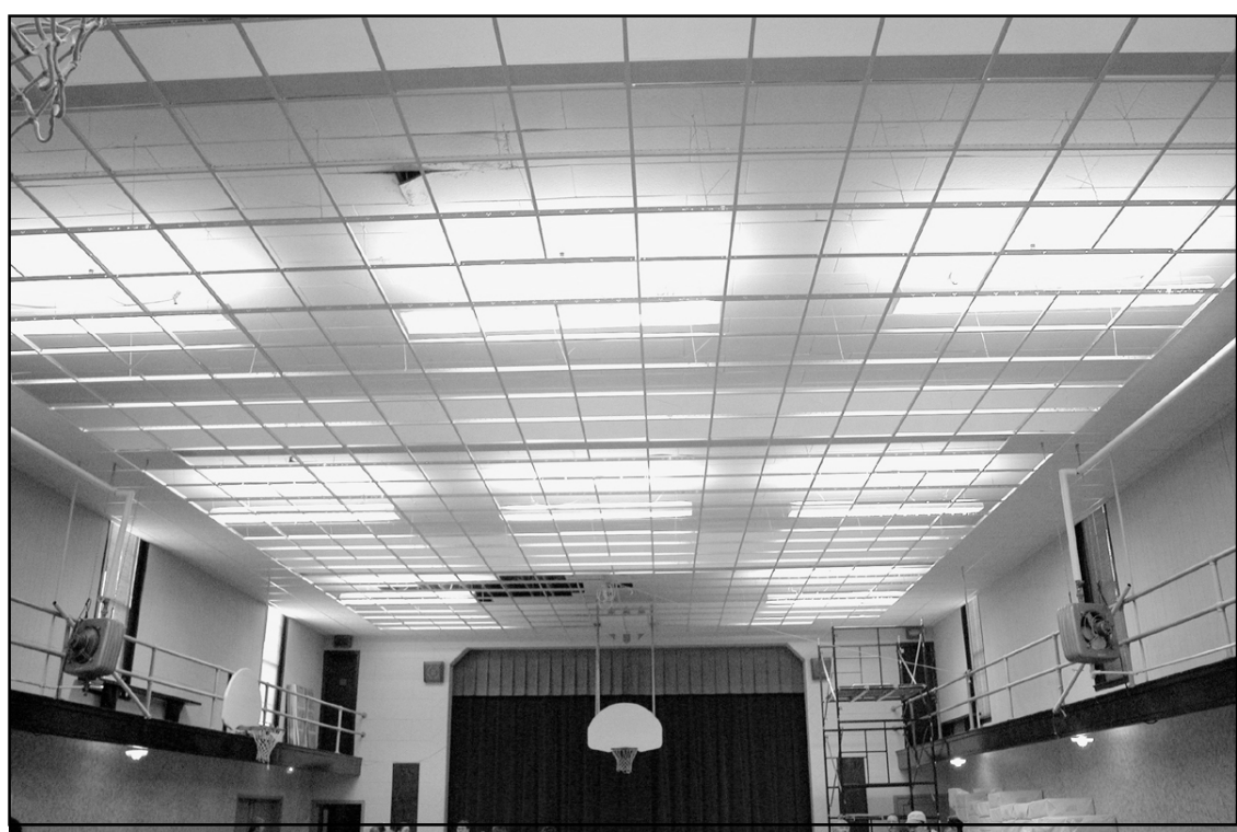
The framework for the new ceiling in the Brandon Auditorium is shown here. The holes were filled with panels and the lights lowered.
