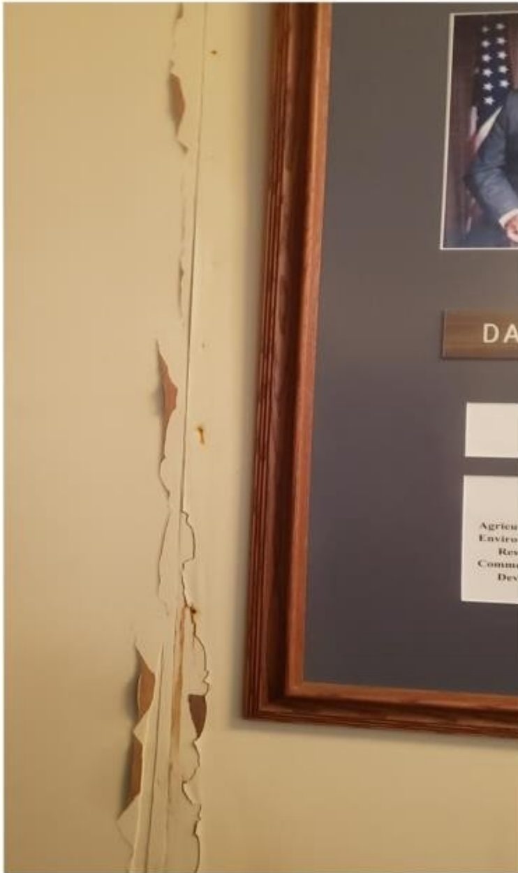
Wallboards Peeling In The Upstairs History Center Display Room
