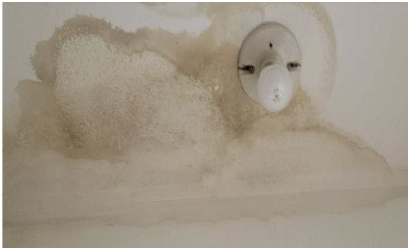
Ceiling in the History Center Closet
